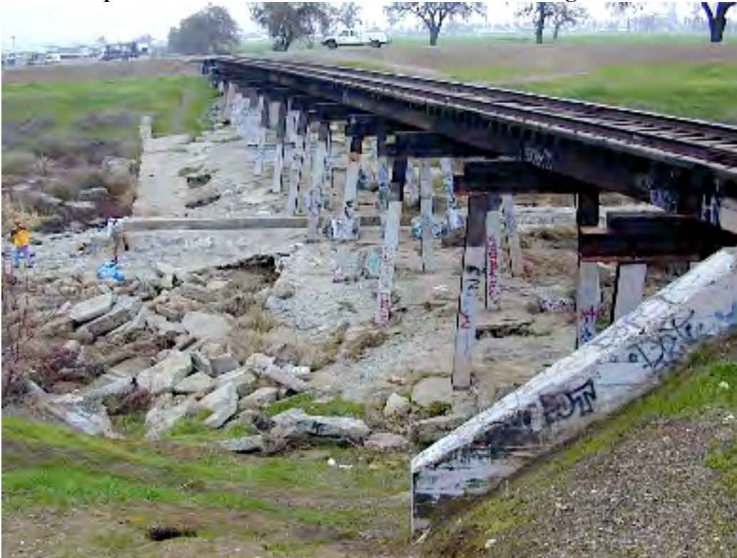
Photo 4. Downstream of Central California Railroad Crossing apron and flume.
