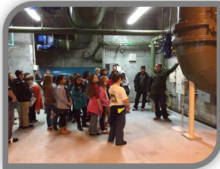
Water Operations Manager Jim Wunderlich guides John Muir School's fifth graders through the water treatment process during a tour of the Dr. Joe Waidhofer WTP
