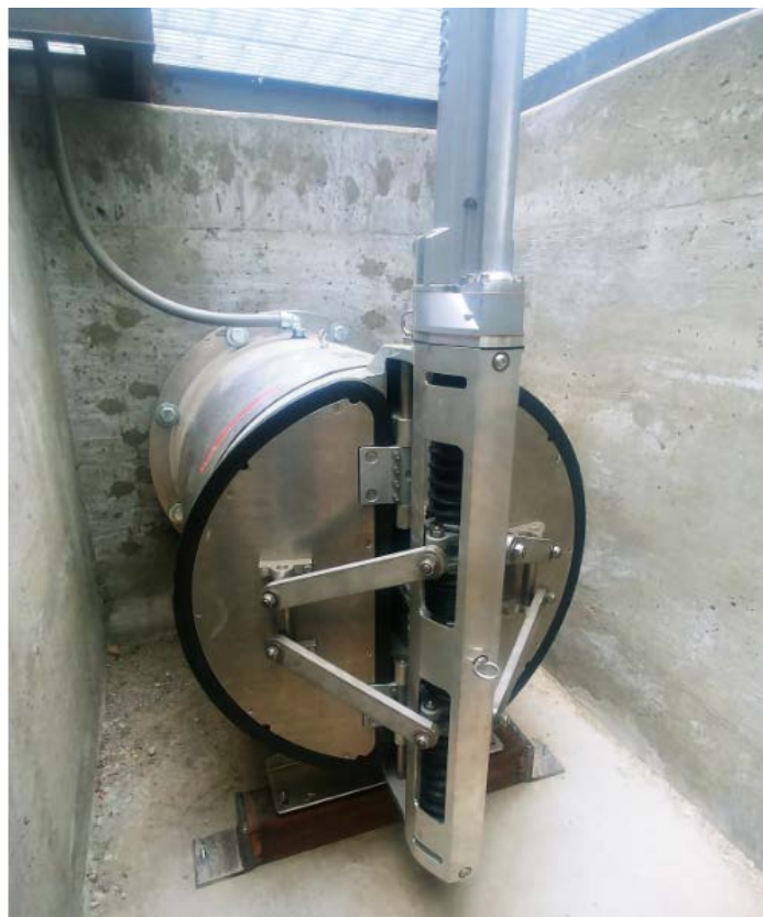
Figure 3-2. Rubicon BladeMeter™ Installed at PC-2.
