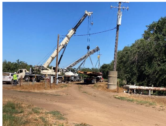
Figure 1 : Power Lines at Gotelli
