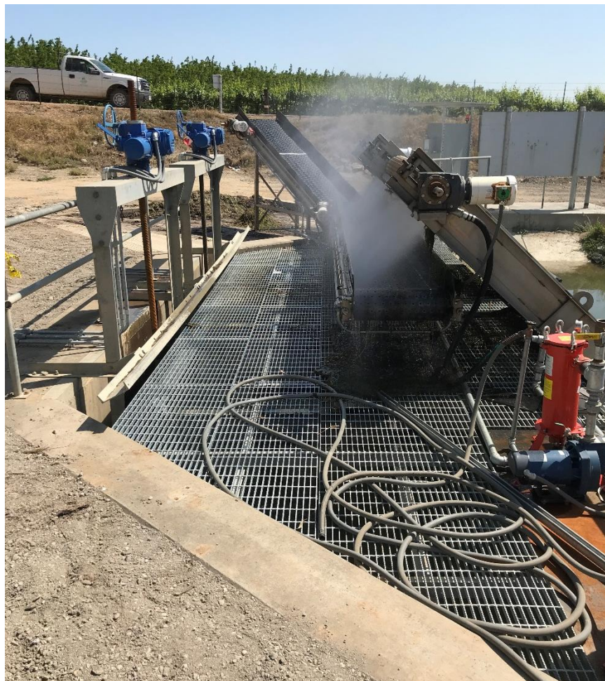
Figure 1 Traveling water screens and conveyor system at Copperopolis Road Gates
