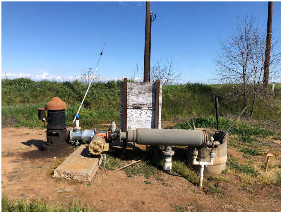
Photo 3. Photograph of existing pump facilities. The proposed slant pumps would be installed to the right (south) of the existing facilities (March 17, 2022).
