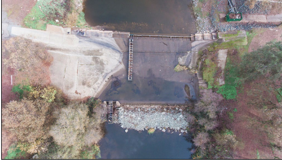
Figure 4.4-4. Overhead view of the Bellota Weir with the temporary fish ladders installed.
