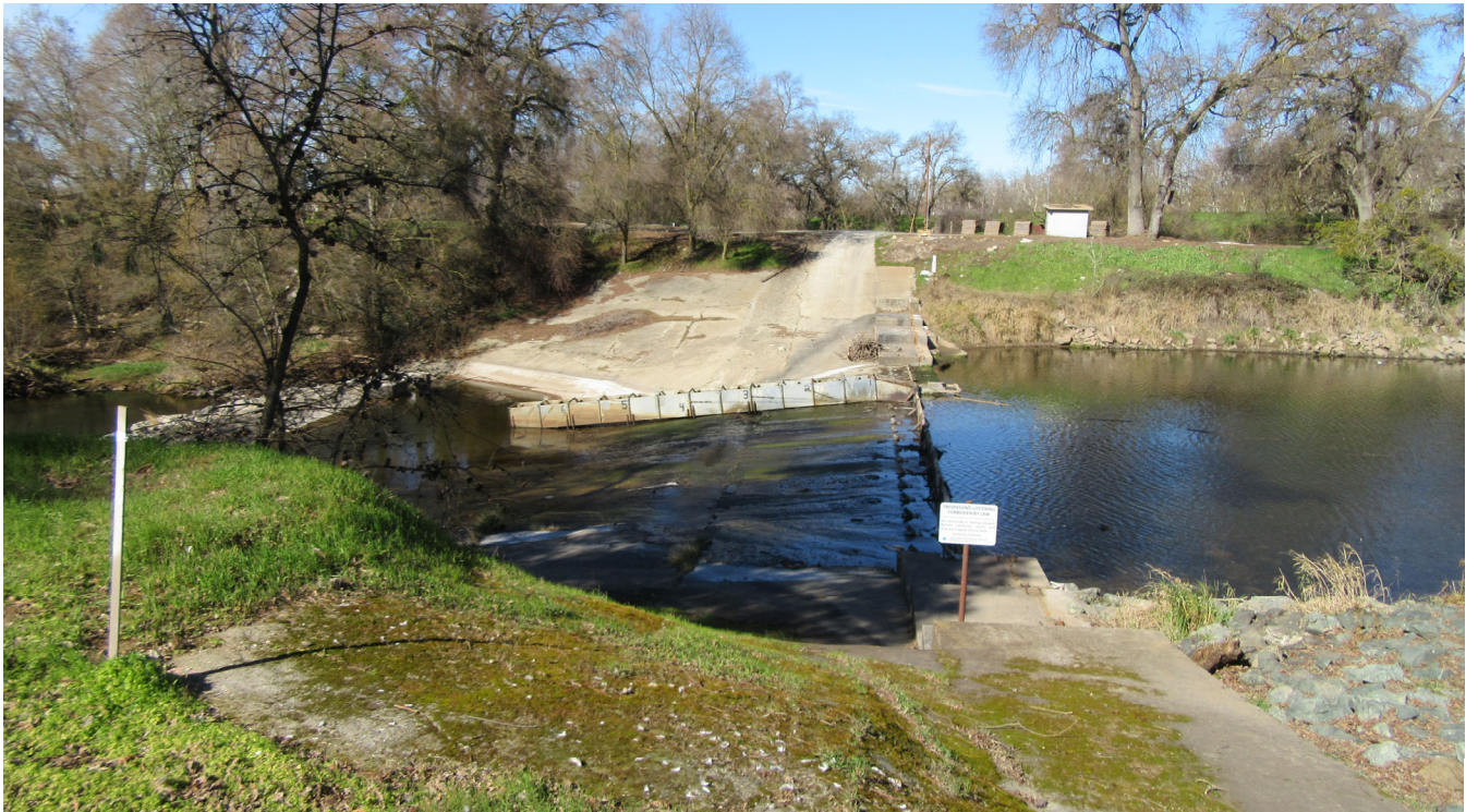
Photo Plate J: Existing Bellota flashboard dam (to be demolished) and fish ladder as viewed from Mormon Slough south bank looking north.
