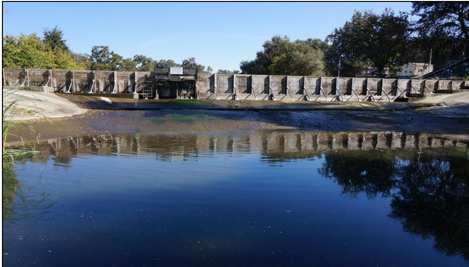
Figure 4.4-3. The 8-ft flashboard dam installed on upstream sill of the Bellota Weir.
