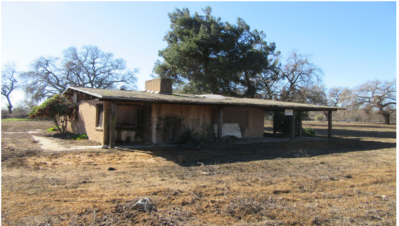
Photo Plate B: Close up of Existing Abandoned Structure to be Demolished looking west
