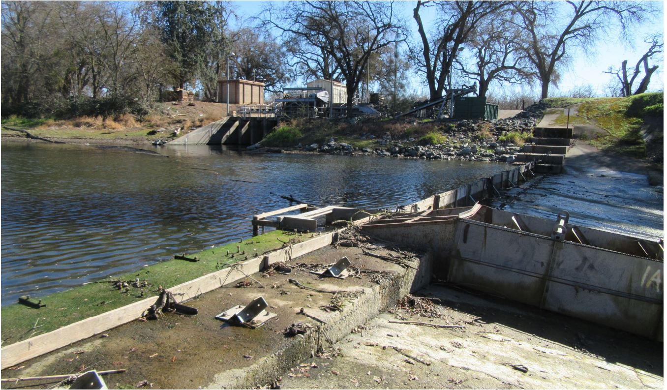
Photo Plate I: Existing Bellota flashboard dam (to be demolished) and fish ladder as viewed from Mormon Slough north bank looking south. Existing Bellota intake structure and trash rack operations in background. Existing small structures shown on Photo Plates G and H are visible in the background beyond the intake.
